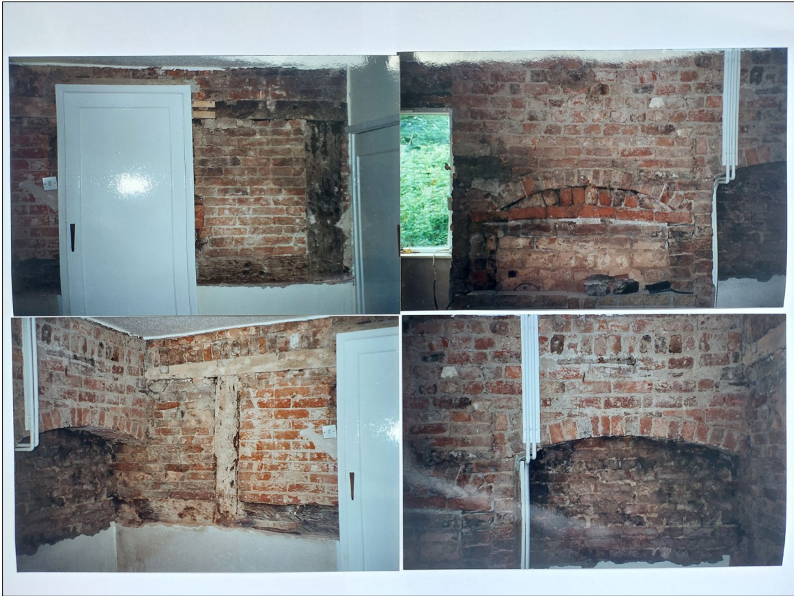
Figure 124: Interior of No. 10 The Green, the former Pipe and Punch Bowl public house.
